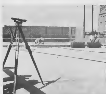
TO INSURE level placement of forms and screeds, a theodolite serves as constant reference. Into the forms, complete with reinforcing rods, is poured the concrete, about 3 1/2 cubic yards at a time.
